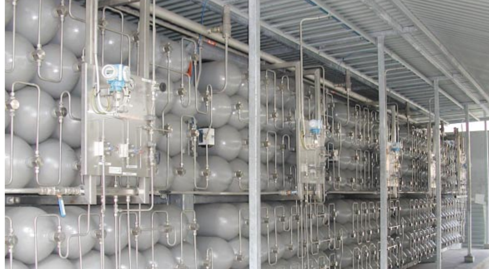
Cylinders are used for storage of pressurised biogas to even out differences in production and use.
