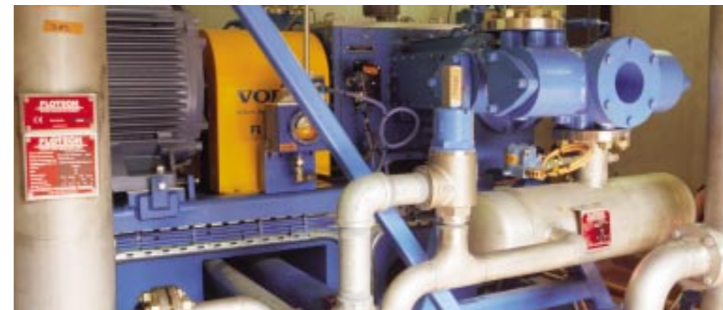
The combined production of heat and electricity means that the energy contained in the biogas is most efficiently utilised.
