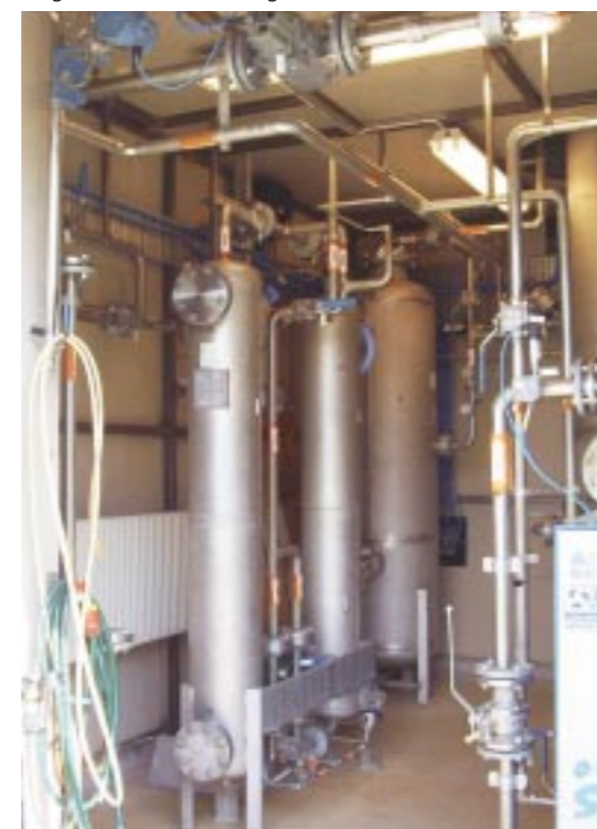
Biogas is dried before being used as a vehicle fuel.
