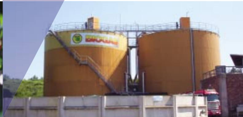
In a biogas process, microorganisms degrade organic waste into simple components. This process is completely anaerobic, that is without any contact with oxygen. Nutrients are concentrated in the residue, whereas almost all the energy is conserved in the final product, methane.
